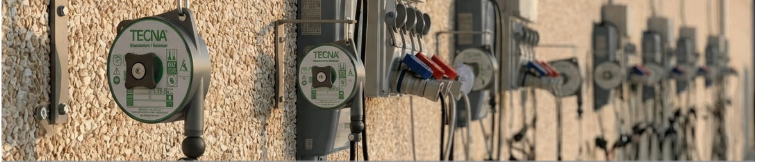
Electric Pallet Truck Charging • Forklift Fleet Charging
