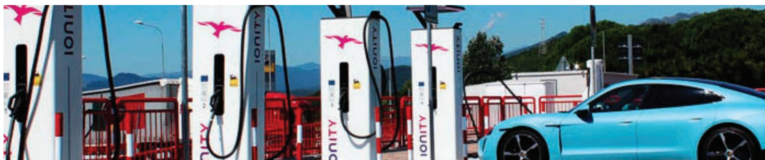
HPC EV Charging • Commercial Parking Charging
