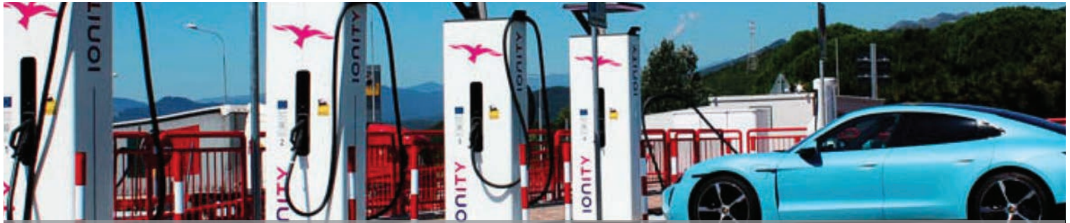
HPC EV Charging • Commercial Parking Charging
