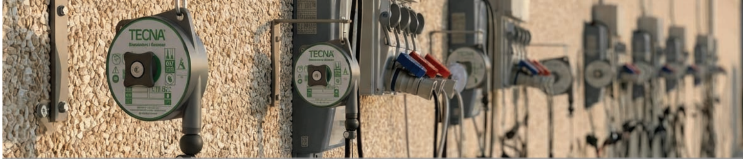
Electric Pallet Truck Charging • Forklift Fleet Charging
