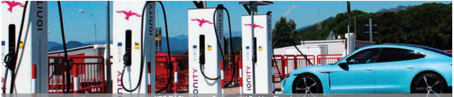
HPC EV Charging • Commercial Parking Charging
